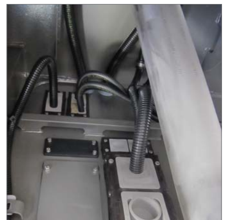
KEL-JUMBO 2 - Page 48 / KEL 24|x - Page 16 Routing of conduits and large cables in the vehicle frame.
